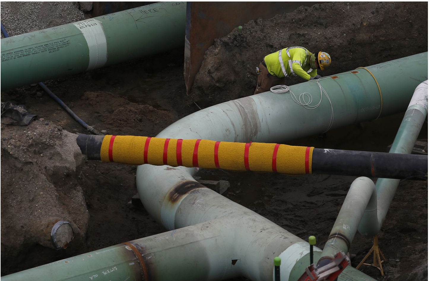
A construction worker bent down next to a pipe on the Enbridge compressor worksite. JESSICA RINALDI/GLOBE STAFF
