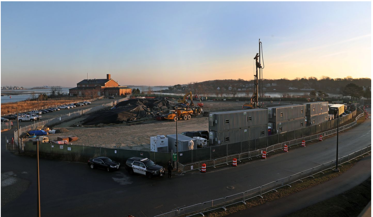
This past January, workers began construction of the 7,700-horsepower compressor, which would pump gas under high pressure to speed its journey north, as far away as Nova Scotia. DAVID L. RYAN/GLOBE STAFF
